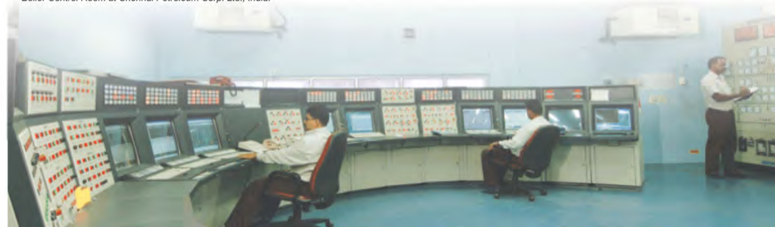
Boiler Control Room at Chennai Petroleum Corp. Ltd., India.
