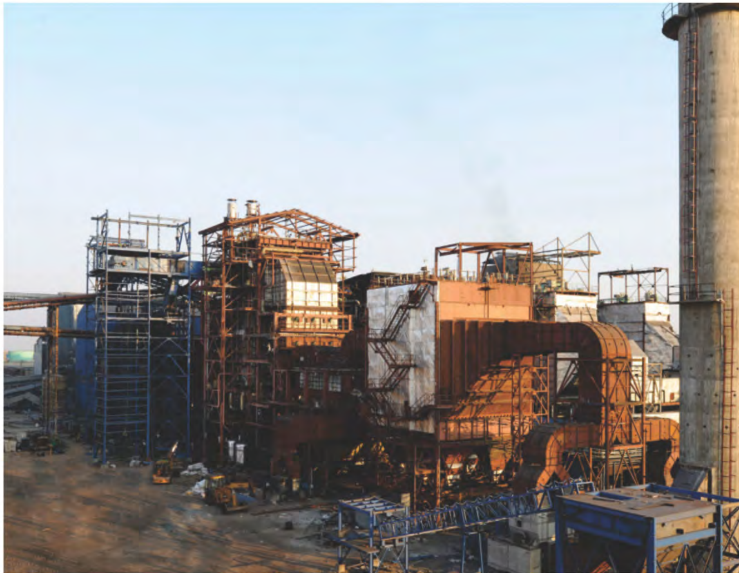
30 MW Cogen Power Plant on EPC basis including civil work for Shree Renuka Sugars Ltd., India.
