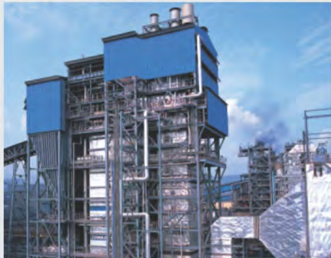
150 TPH CFBC Boiler with Compact Separator for Jindal Steel & Power, Raigarh, India.
