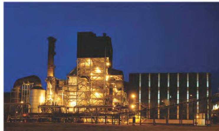
30.4 MW Complete Cogeneration Plant supplied on EPC basis to Zambia Sugar Plc. (a subsidiary of Illovo Group of South Africa) Nakambala, Zambia.
